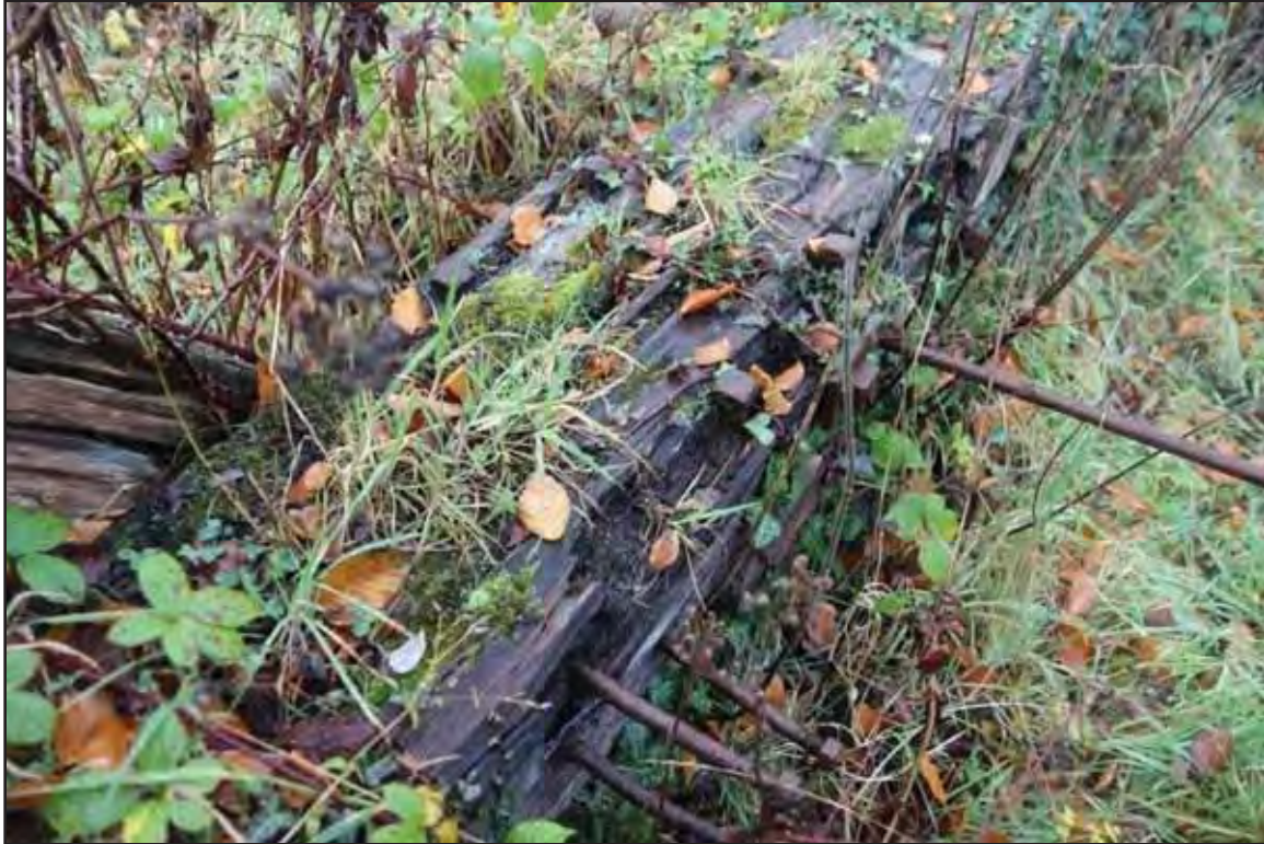
Photo 4 - Main Sliding Timber - Severe Rot
