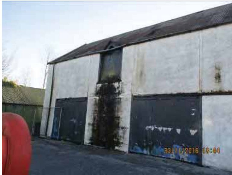
Photograph 8 View of shed openings with clear signs of continuous water damage from the first floor opening.
