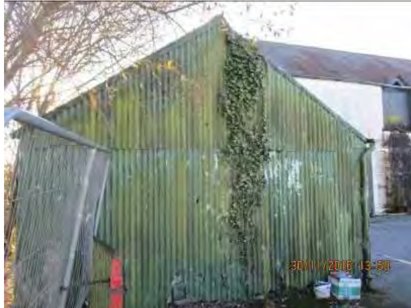
Photograph 9 View of gable end of corrugated iron shed with holes visible in the sheeting.
