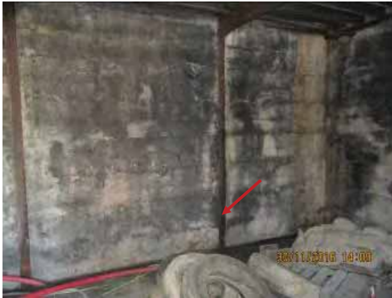
Photograph 4 View of building interior with wasted column base highlighted
