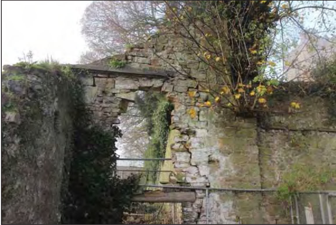
Photo 2 - Damaged Corner of Cathedral Wall
