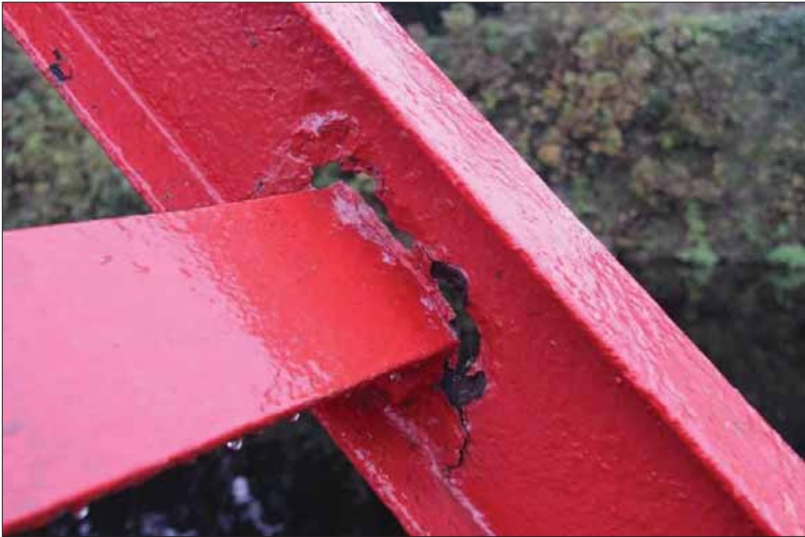
Photo 7 - Necessary Structural Repairs to Ironwork
