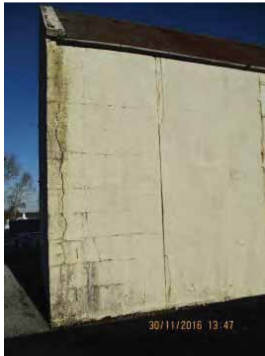
Photograph 7 View of patent crack defect.
