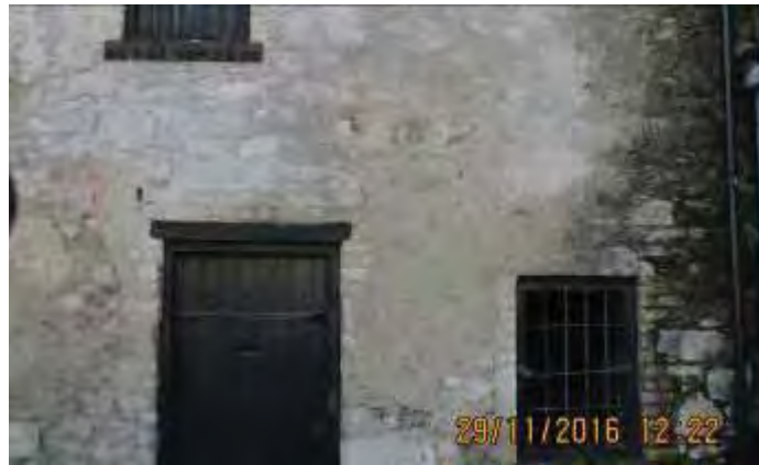
Photograph 5 View of remnants of original render
