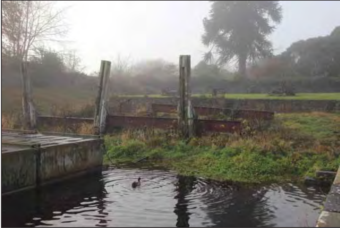
Photo 8 - Upright Sections in Poor Condition
