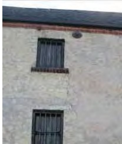
Photograph 3 Vertical crack between 1 st and 2 nd floors
