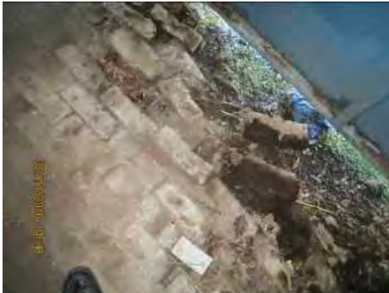
Photograph 5 View of wooden block floor with loose blocks on view.
